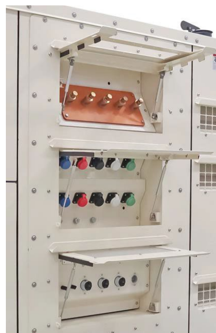
Distribution panel (side)
