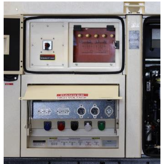
Distribution panel (side)
