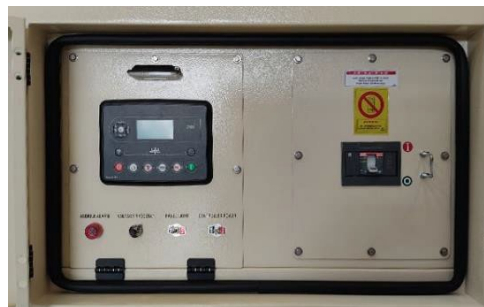
Control panel and breaker (rear side)
