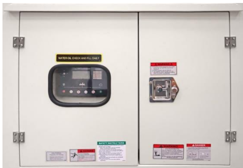
Control panel and breaker (rear side)
