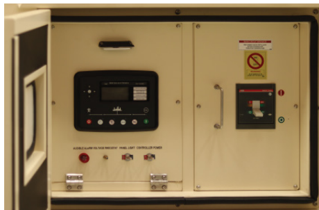
Control panel and breaker (rear side)
