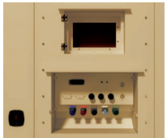
Distribution panel (side)
