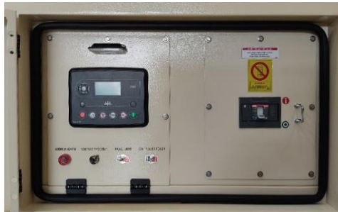
Control panel and breaker (rear side)
