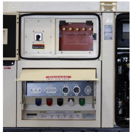
Distribution panel (side)
