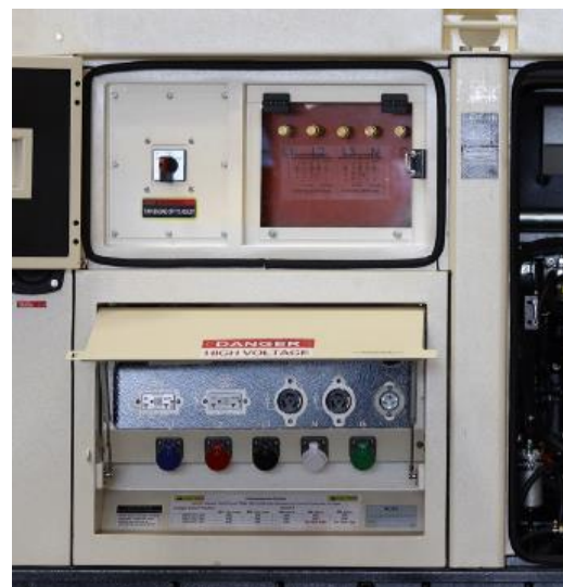
Distribution panel (side)
